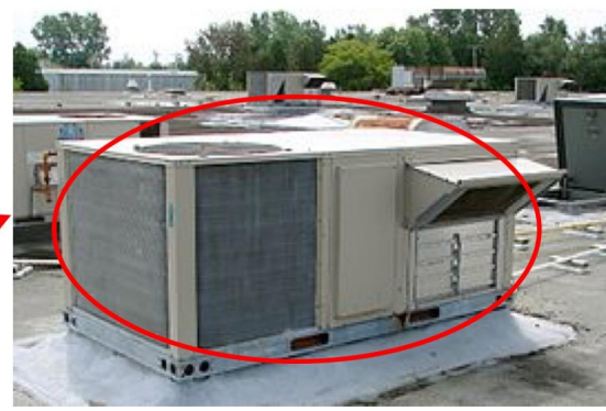
Air handling unit
